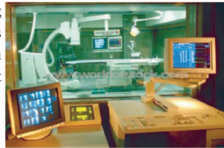
Figure 1.34. Hospital with Life saving computer controls
